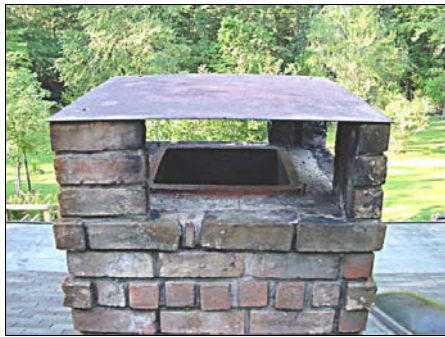
Capped chimney that is still accessible to Chimney Swifts Photo by Tee Tarlton
