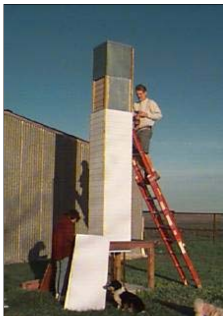
Installing insulation and a second skin on the Mc5 tower near Lockhart, TX
