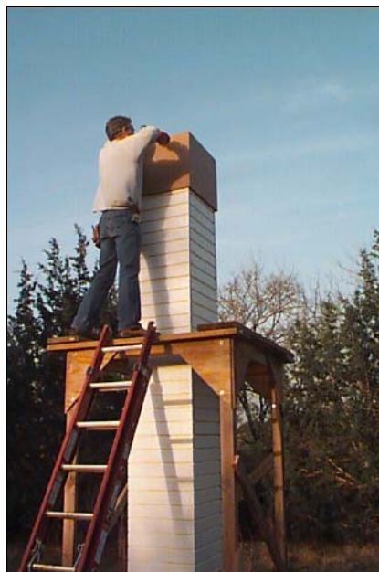
Installing insulation, a second skin and new predator guard on the Jandarosa Tower Photo by Georgean Kyle
